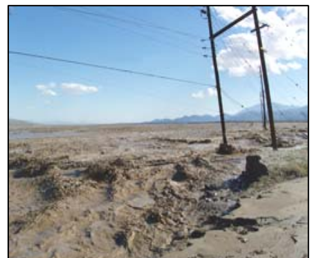
Flooding along Indian Canyon Drive, January 11, 2005.
