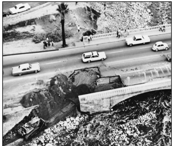
Flood damage to Highway 111 from 1965 storms. (Source: RCFCWCD)
